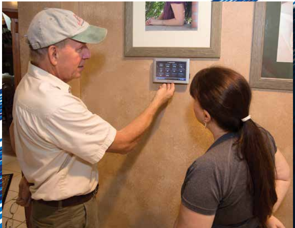
Efficient Climate Control owner Paul Stamper explains the workings of the control panel to a homeowner.
